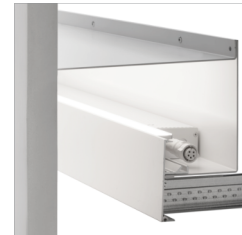
Fixture installed in AXIOM Classic-Edge cove
